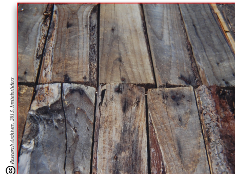
The same challenges faced by informal builders can be seen in these floor boards, pieced together with worn tools and random materials.
